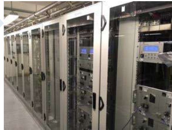
Installed PLC systems in rack room
